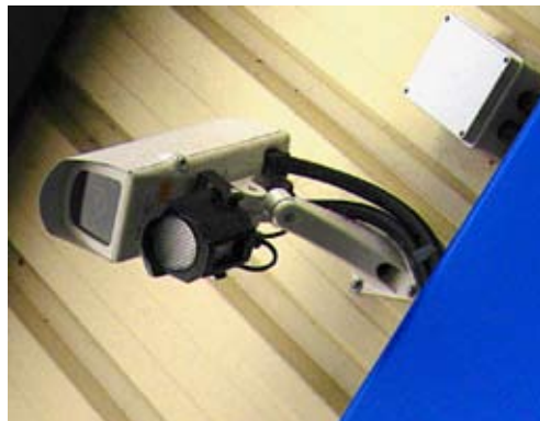
Figure 3.d. IR-sensitive network camera with IR illuminator attached below the camera housing
