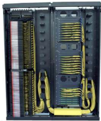
Figure 4. High-Density Optical Distribution Frame
